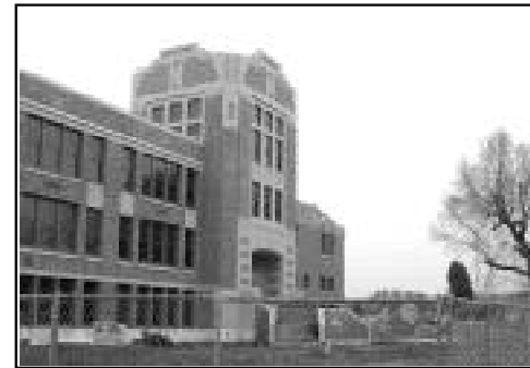
Removal of the old middle school wing is complete. Construction continues at Renton High School
